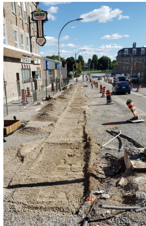
Grading for Concrete Curbs from Main to Chambers can be seen in this photo.
